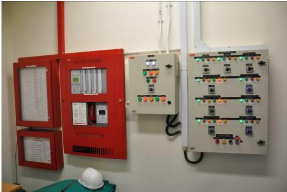
Main Fire Alarm Panel
